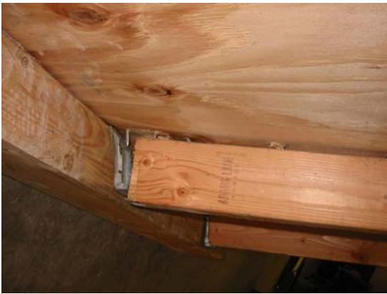
Separation of Strap from 2x4 Subpurlin Photograph 5
